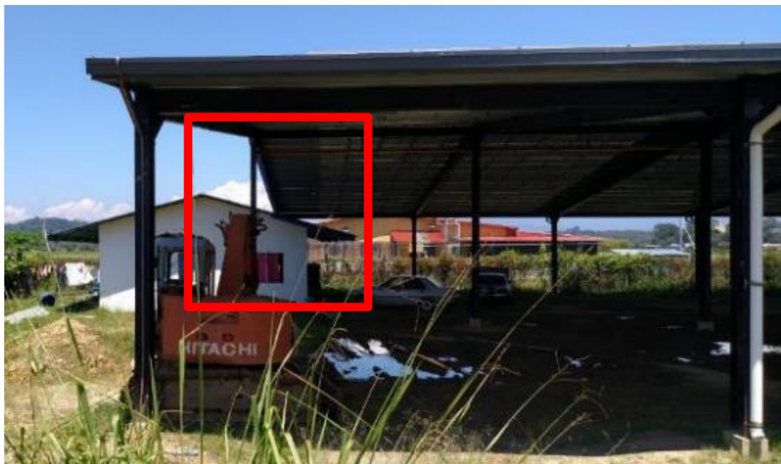
Figure 14 - Overlapping Of PV Roof On Top Of An Existing Roof
