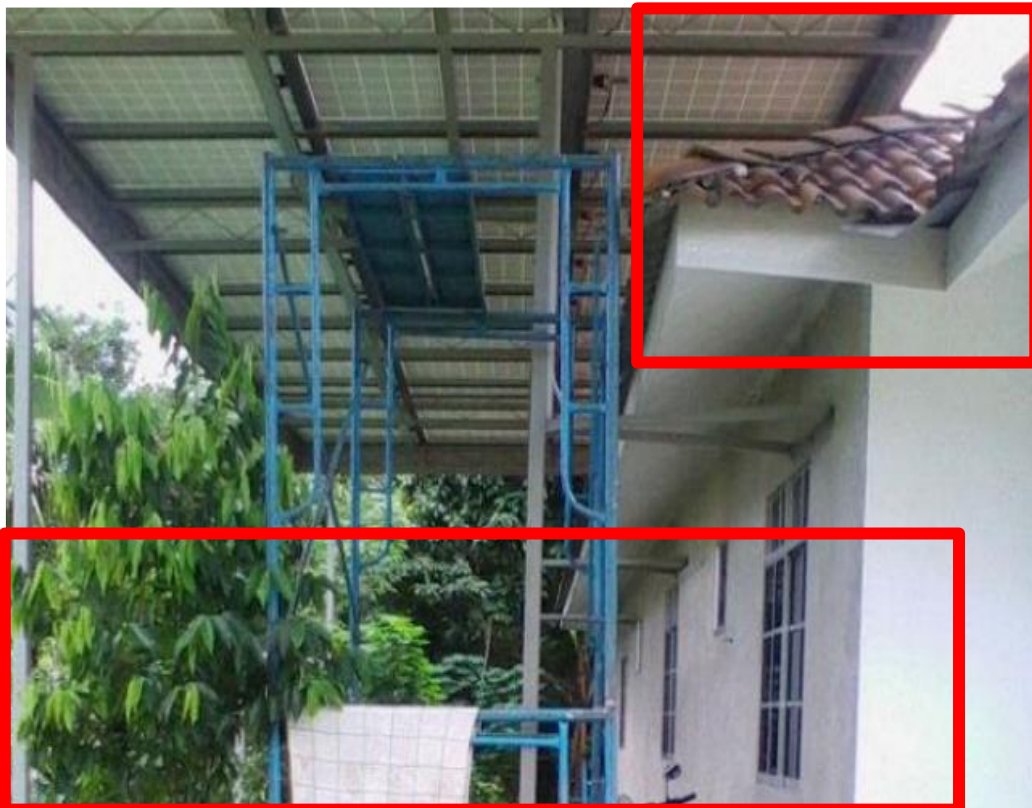
Figure 11 - Overlapping Of Modules On Top Of Existing Roof & Using Inappropriate Construction Materials
