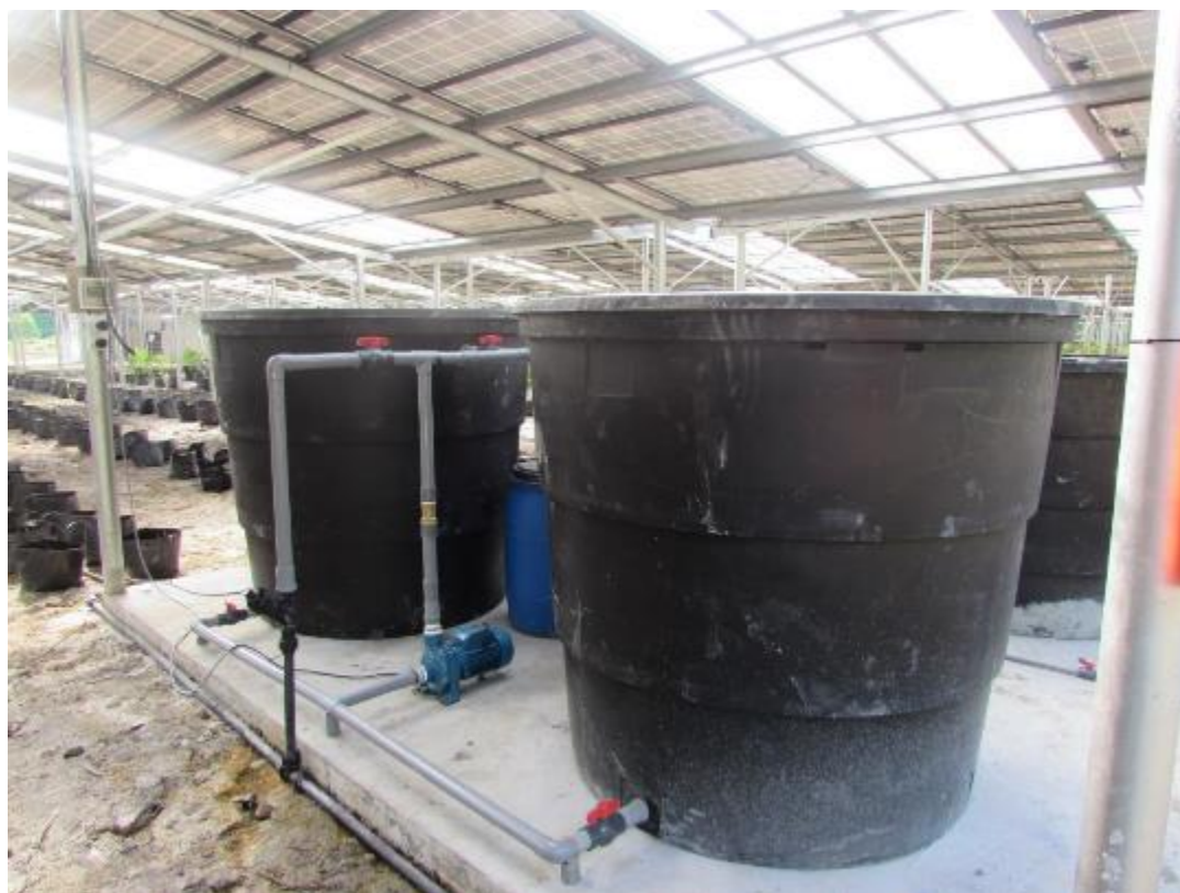
Figure 25 - Rain Water Harvesting Constructed And Used For Agriculture/Aquaculture
