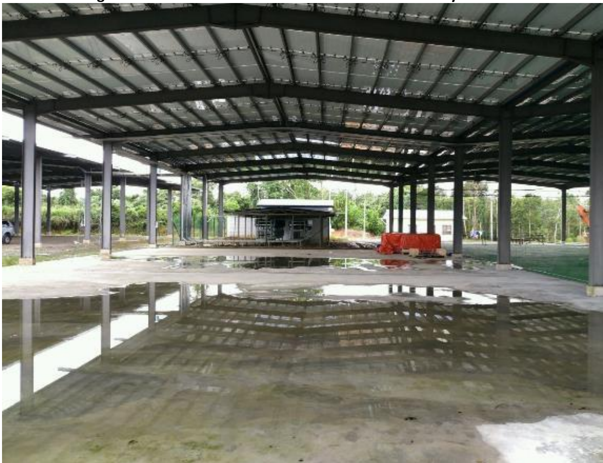
Figure 33 - The Ground Below The Structure Is Not Fully Utilized (And Concrete Floor Is Wet Maybe Due To Roof Leaking)
