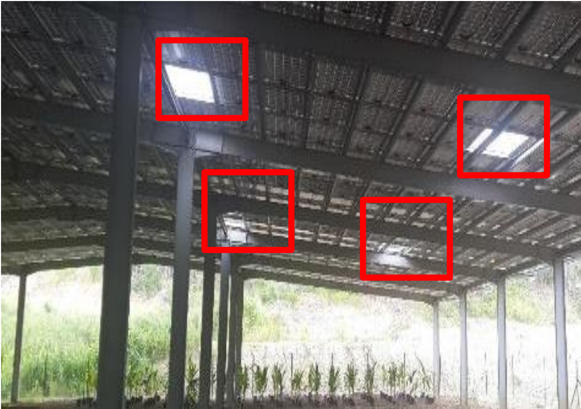
Figure 15 - All PV Arrays MUST BE COVERED. Sunroofs Can Be Installed To Allow Penetration Of Sun.
