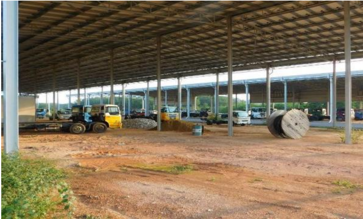
Figure 32 - The Ground Below The Structure Is Not Fully Utilized
