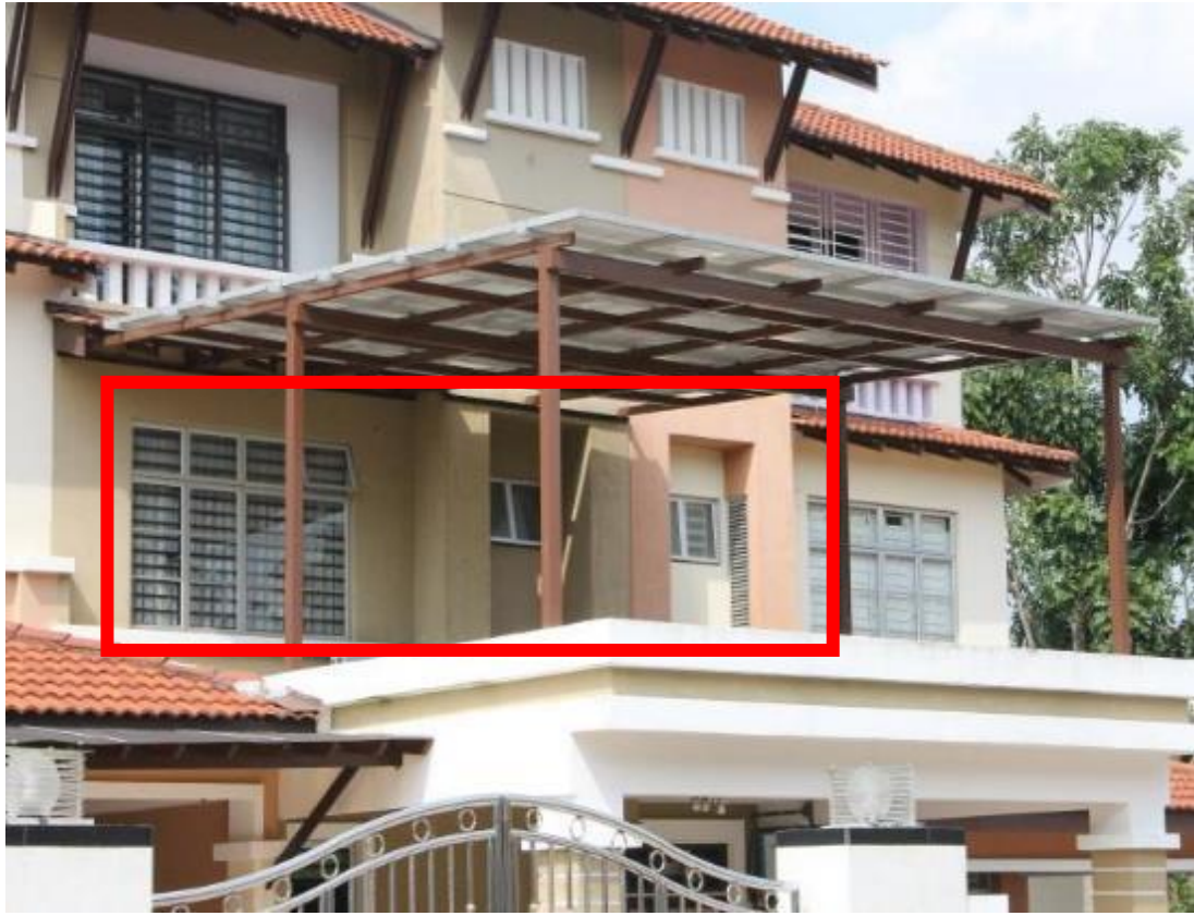
Figure 8 - No Access Door As To Serve The Function Of Installation As A Balcony
