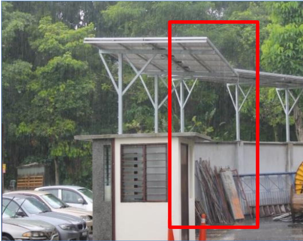
Figure 17 - Installation serves no function or purpose(Walls Do Not Need Roof)
