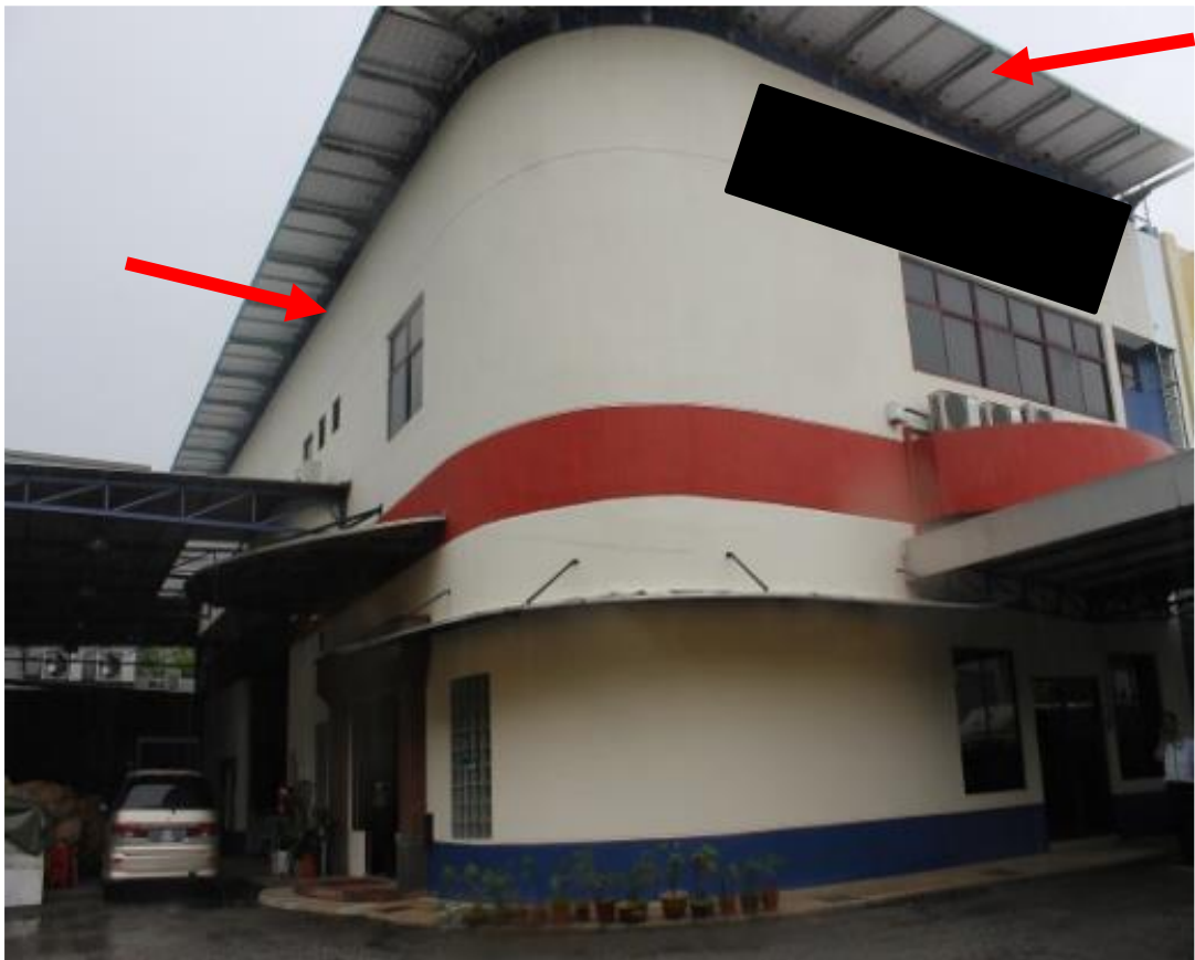
Figure 16 - Installation serves no function or purpose (PV Module Too High to Serve as Roof)
